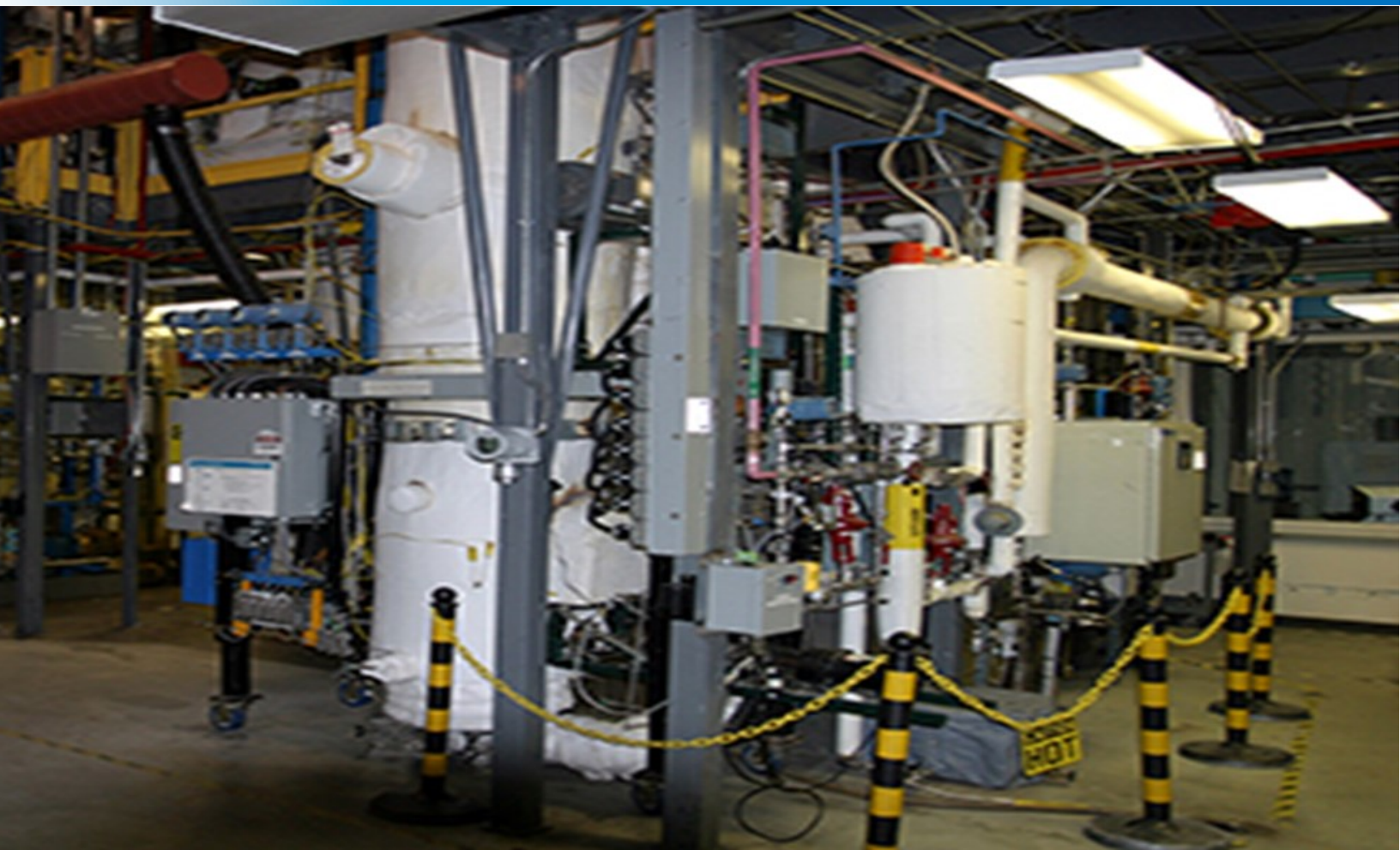
Fig.3 This Thermochemical Process Development Unit at the National Renewable Energy Laboratory (NREL) can pyrolyze biomass into bio-oil for conversion to hydrogen. Photo from NREL
