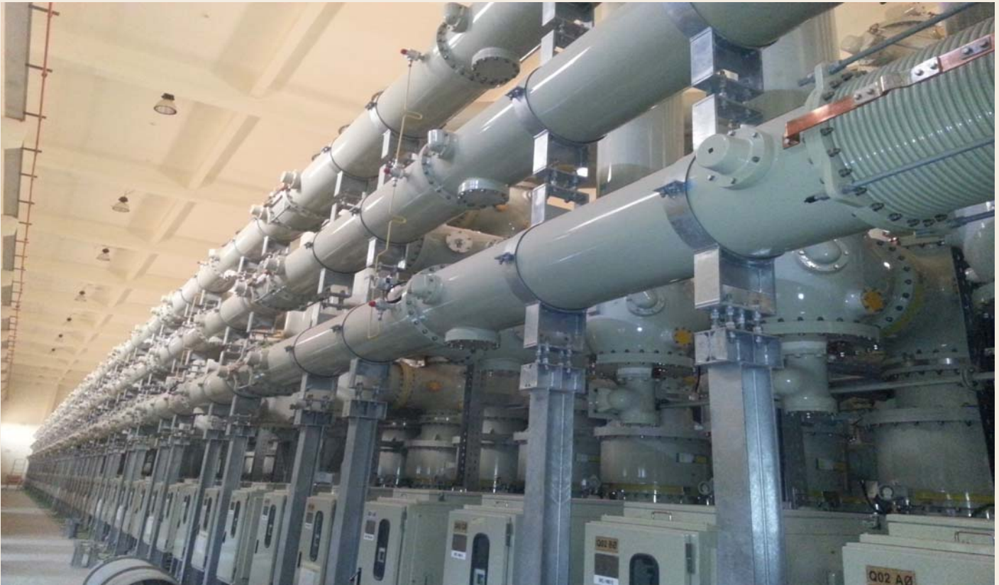
Giza North 500 kV GIS
