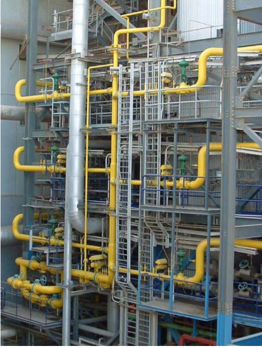
Fig. 1 Control valves in SIDI KRIR Power Station
